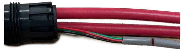
Appendix Figure 3: Installed into cable gland fingers with .787 in [20mm] measured and marked from back of insulation
